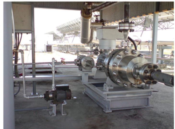
Hermetic Canned Motor Pump in operation in Spain at the Plataforma Solar de Almeria (PSA), pumping water 300°C with 100bar system pressure (Image courtesy of Auquime SA)
