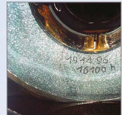
Suction-side wear plates of the same absorber circulation pump after an operating time of 16,000 hrs. each
