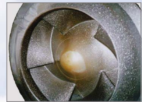
Impellers of two absorber circulation pumps after an operating time of 11,000 hrs. (left) and 24,000 hrs. (right) in the same operating environment
